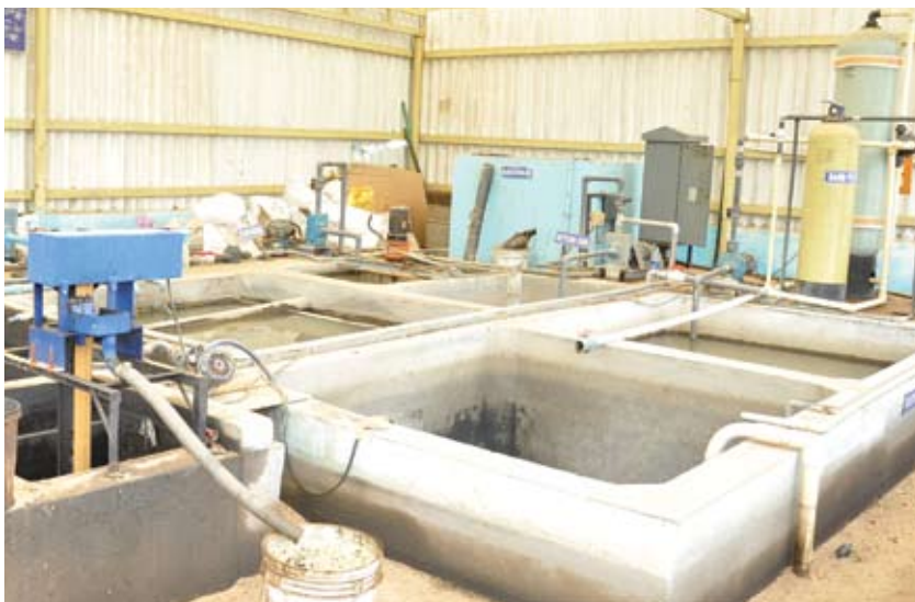
Effluent Treatment Plant at Nandi Toyota
