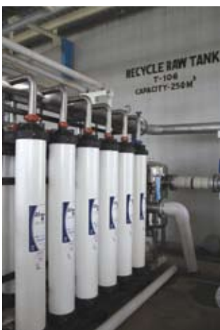
Reverse osmosis unit
