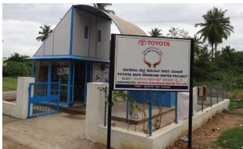
Water purification unit installed at Byramangala village
