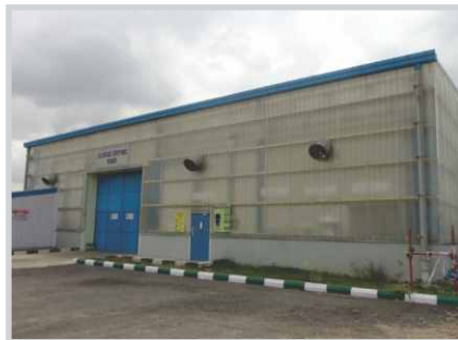
Sludge yard based on solar Greenhouse effect
