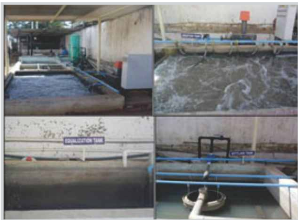
Wastewater Treatment System at Nandi Toyota, Bangalore
