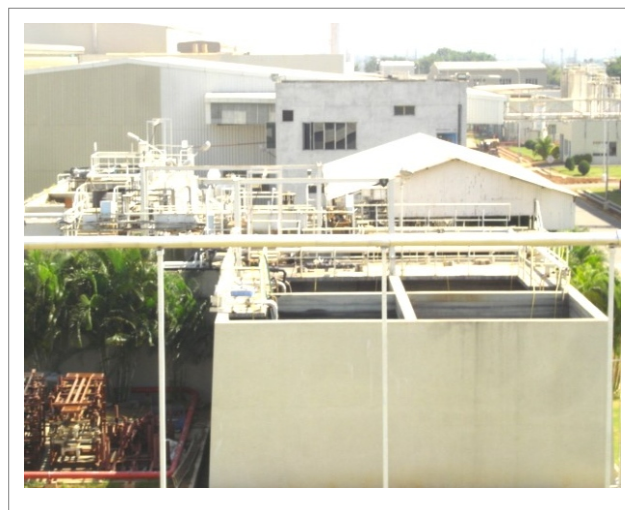
Fig 6 : TKM Wastewater Treatment Plant
